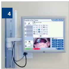
4 Remote Touchscreen Near Circulator Desk
